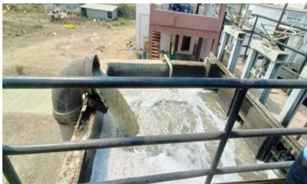
Fig - 5: Initial Condition of Sewage Water
