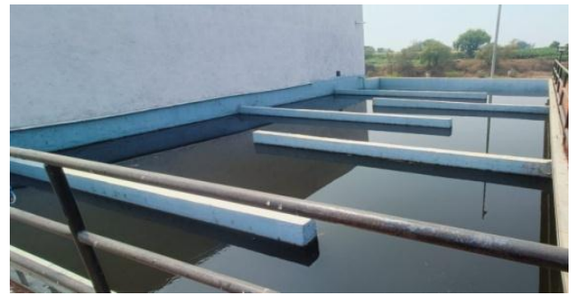
Fig - 6: Final Condition of Sewage Water
