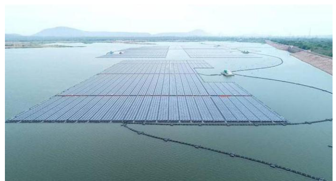
Figure 1 100 mw floating solar power plant at Ramagundam, Telangana
