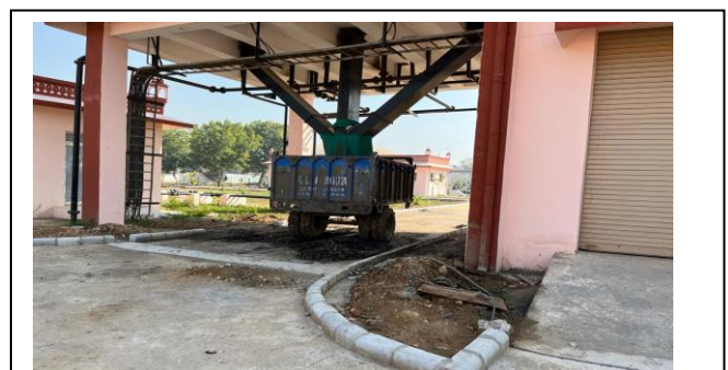
Fig. 1. Photograph of - Sludge collection at Dehalawas STP, Jaipur
