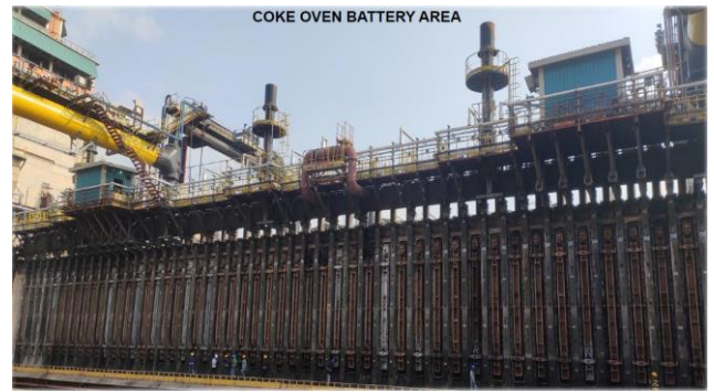
Figure 4 Coke Oven Batteries
