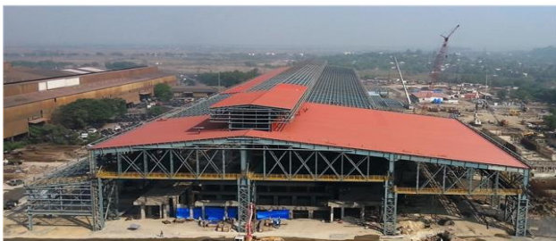
Figure 8 Typical Steel Bar Mills
