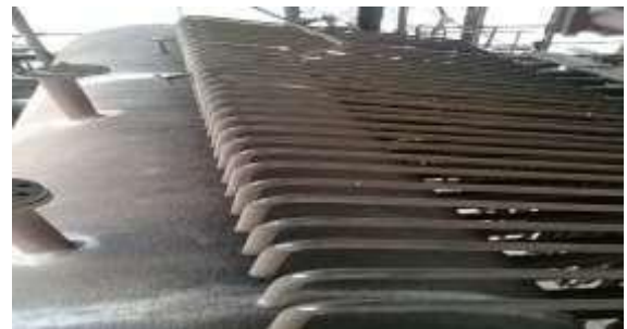
Fig.1.1 Actual photograph of Steam drums of a super heater
