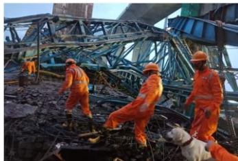
Fig 3: Thane crane accident
