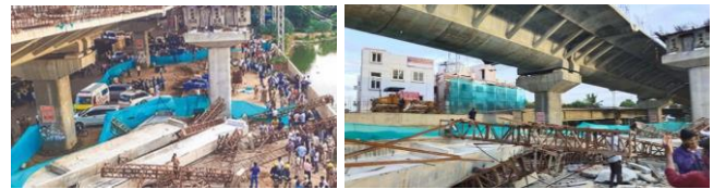
Fig 1: Natham flyover collapse
