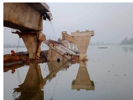
Fig 2: Kollidam bridge collapse
