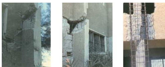
Figure-2 Damaged elements
