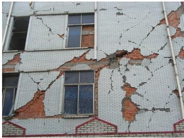
Figure-6 Damage of RC building with masonry infill
