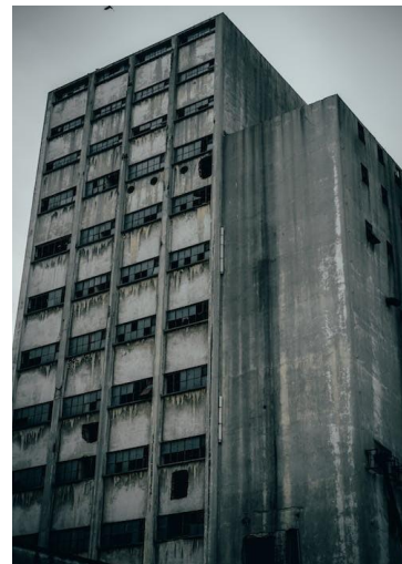
Figure-1 Old Damaged Building
