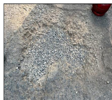
Fig- 8: Pothole Covered with Aggregate
