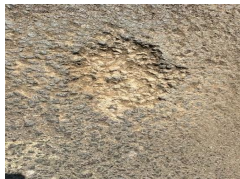
Fig-13: Before Filling the Pothole
