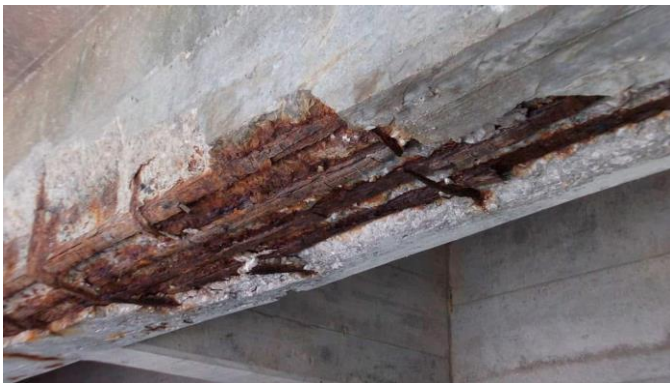
Fig -1: Corrosion of RC beam [16]
