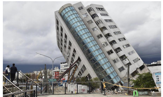
Fig.1: Collapsed Building Due to Earthquake
