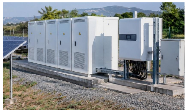
Figure 2. Closer view of battery storage cabinets and associated equipment.
