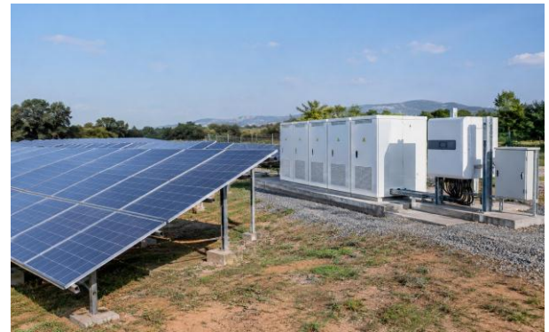
Figure 1. Solar PV panels integrated with battery energy storage equipment.
