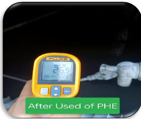
Fig.3 Temperature reading of water after using PHE
