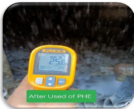
Fig.4 Temperature reading of water in the running condition of condenser
