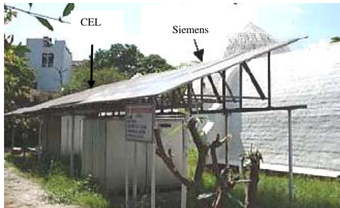
Fig.1: Stand- alone Solar PV array system setup at IIT Delhi, India
