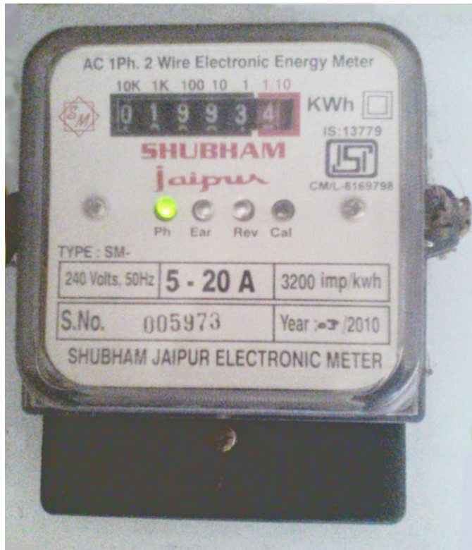
Fig-2: Single phase analog energy meter
