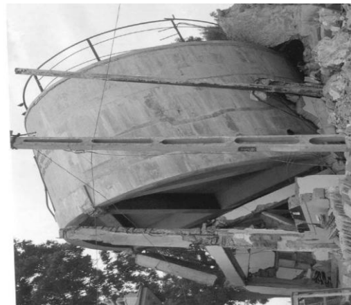
Fig-1: Collapsed Slender and Weak Framed Staging of Water Tanks in Bhuj Earthquake
