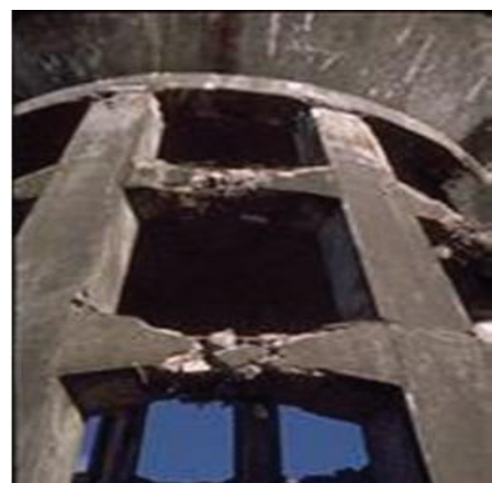
Fig-2: Bending-Shear Failure in Beam
