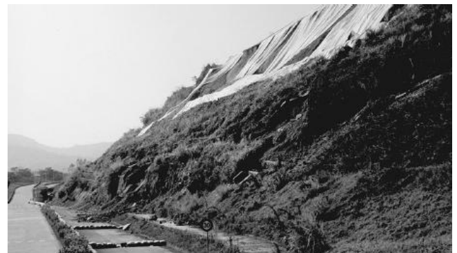
Fig -1: Side view of reinforced slope failure due to Chi-Chi (Taiwan, 1999) earthquake
