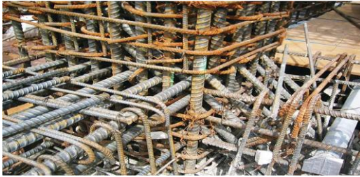
Fig. 2 Congestion at the Beam-Column Joints (ref.: www.concreteconstruction.net )
