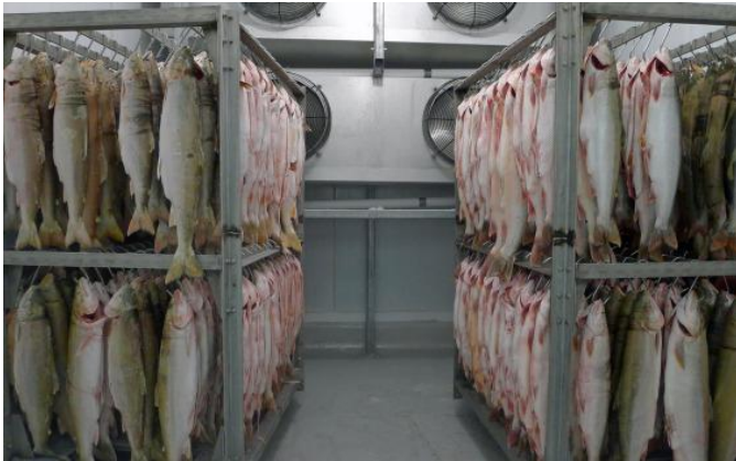
Fig.1: Air Blast Freezer
