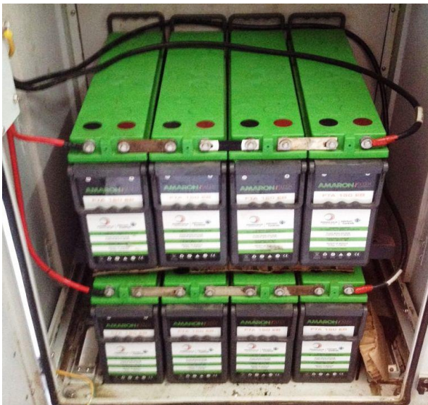
Fig-16: Battery Strings (Power Backup/DC Storage Systems)
