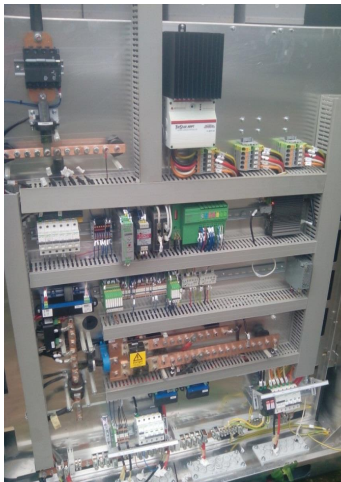
Fig-21: A physical view of Flexenclosure e-site Equipment
