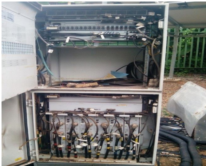
Fig-4: BTS for Out-Door Site
