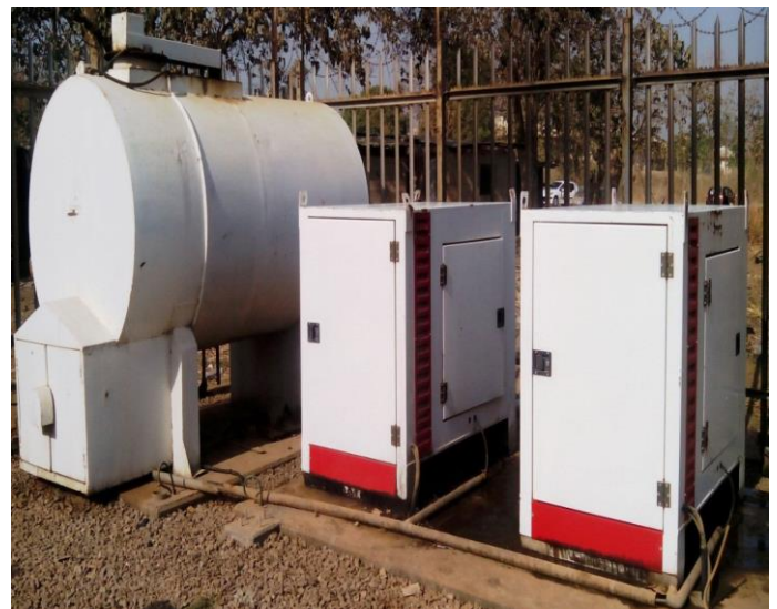
Fig-9: Typical AC Generators on a Telecommunication Site
