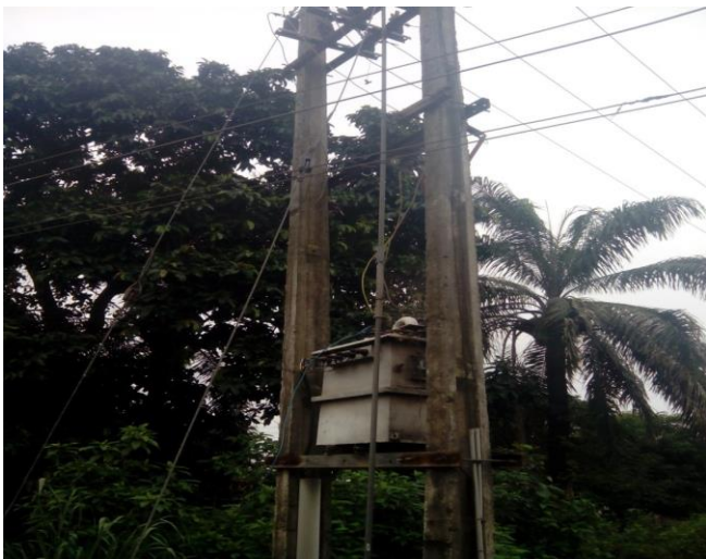
Fig-7: 100kva Transformer for Commercial AC supply to Telecommunication Sites
