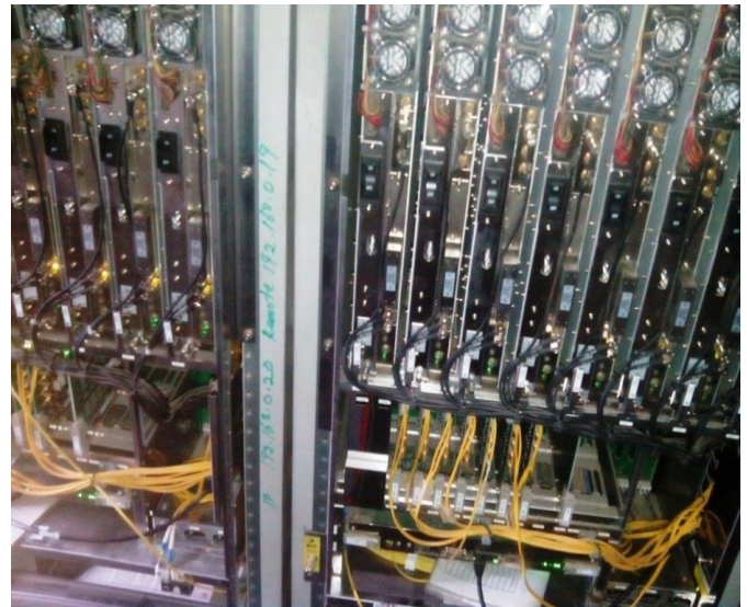
Fig-6: Transmission Radios of a BTS
