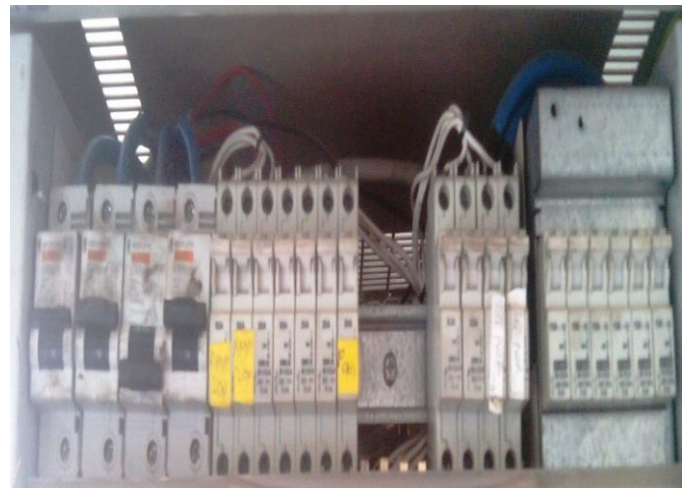
Fig-18: DC Distribution board of Rectifier system equipment
