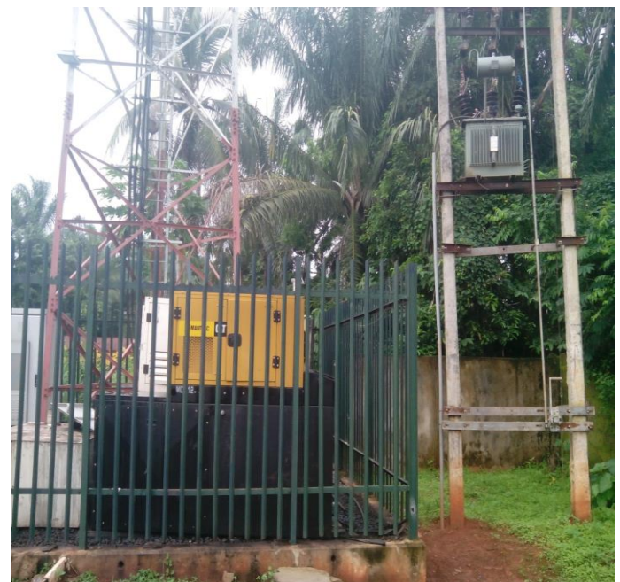
Fig -1: A typical View of a Telecommunication Site/complex in Nigeria.
