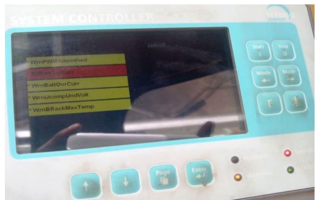
Fig-19: A typical overview of a Generator Alarm
