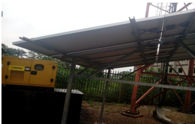
Fig-20: A typical hybrid solution (12kw DC generator and 6kw Solar system)
