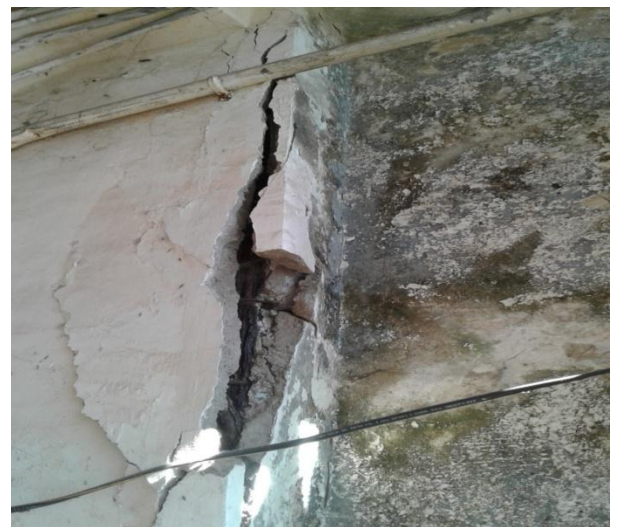
Fig 4.1: Cracks in structural members due to corrosion
