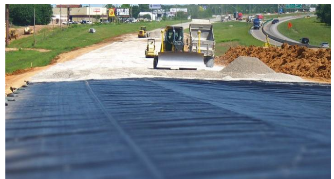
Fig-9: More than 630,000 sq. ft. of geomembrane was installed over expansive clay in Ardmore, Oklahoma to stabilize Interstate 35 [26].
