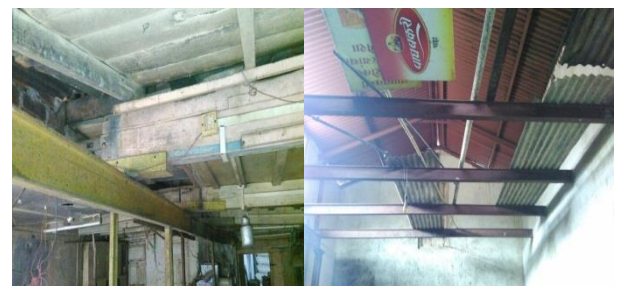
Fig 5 Internal structural condition of Om Prakash Malu Building
