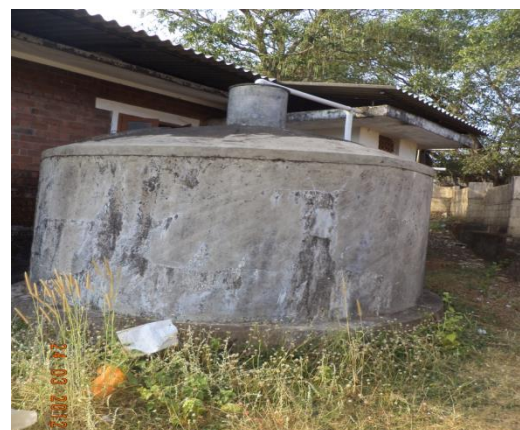
Fig. -3: Roof water harvesting system in the village office, Tavanur
