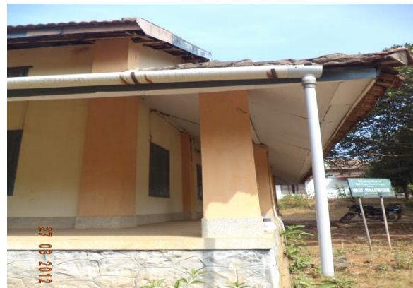
Fig -5: Gutter and conveyance system of RRWHS near library, KCAET, Tavanur
