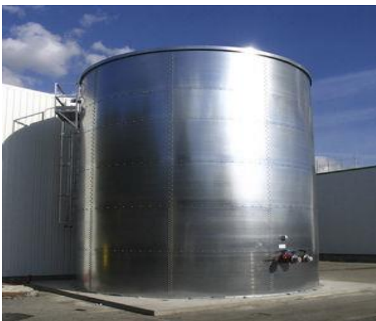
Figure 0.1 Gas storage tank
