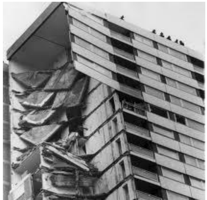
Fig-1: Ronan Point building after collapse, London 1968
