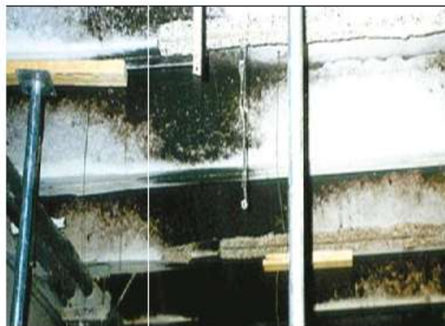
3.1 Separation of Slab & Joist Spalling
