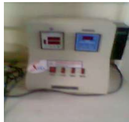
Fig: 5 PID Controller Control box
