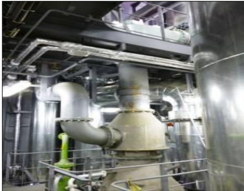
Fig – 6: Deplume reheater unit
