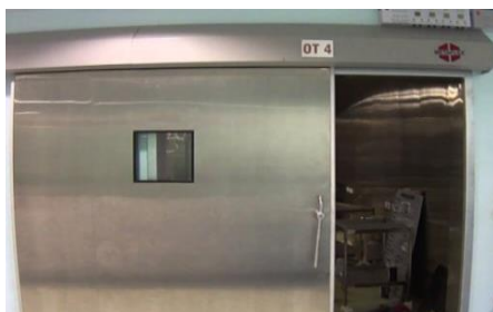
Figure 4- Hermitically sealed door
