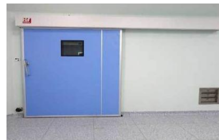
Figure 5- Automatic sealed door
