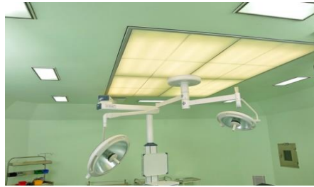
Figure 6- showing ceiling lights of OT.
