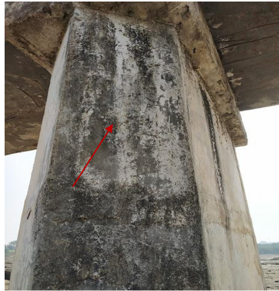
Fig.5 Efflorescence effect over the surface of pier
