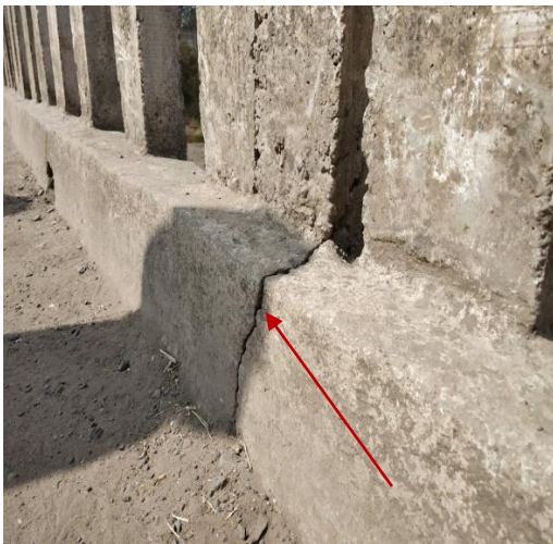
Fig.4 Non-structural crack developed in parapet wall
