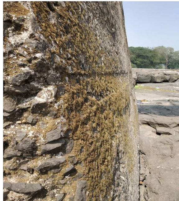
Fig.6 Growth of vegetation over surface of stone masonry pier
