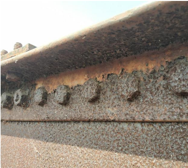
Fig.7 Rusting of the joints of steel truss bridge
