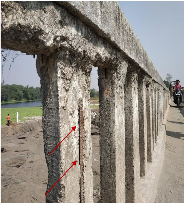
Fig.3 Reinforcement exposed in parapet wall causing decrease in strength in member
