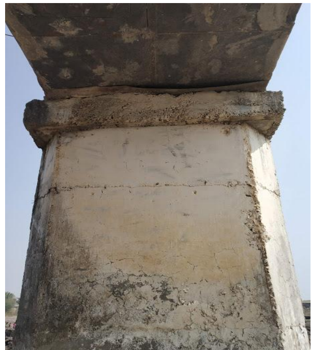
Fig.2 Development of structural crack perpendicular to the axis of pier
