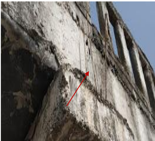
Fig.8 Exposed reinforcement covers of the slab member
