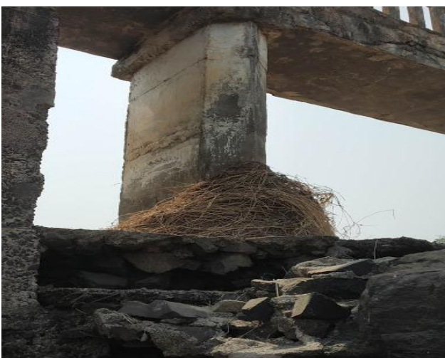
Fig.9 Scouring effect on foundation as well as growth of vegetation
