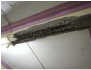
Fig.2.1 Severe corrosion and spalling of beam
