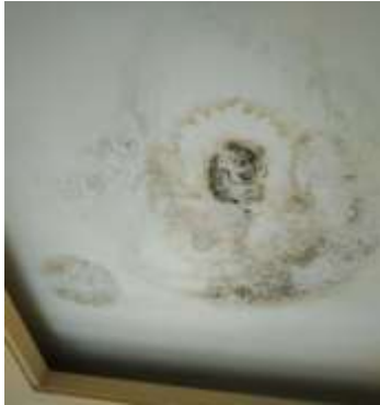
Fig. 2.2 de-lamination of concrete cover due to severe corrosion of roof slab
