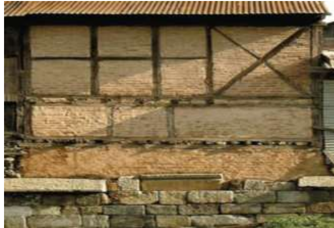
Fig 5: Showing elevation of Dhajji-Dewari Construction in Down-Town Srinagar (Source: 'Randolph Lagenbach book-Do not tear it down').
