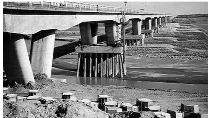
Fig (1) scour around complex piles
