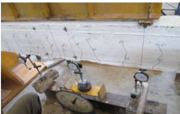
Fig.5 Crack Pattern of RC Beam
