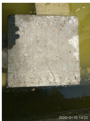
Fig - 6 : Self Repair of Crack
