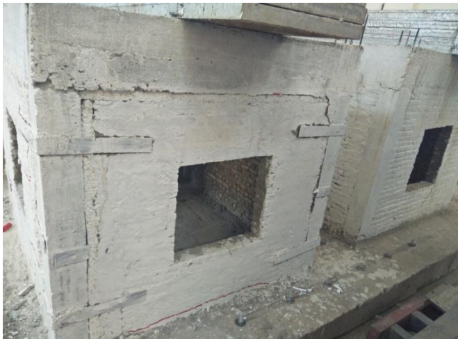
Figure 6: Cracks at 100% of NR2
