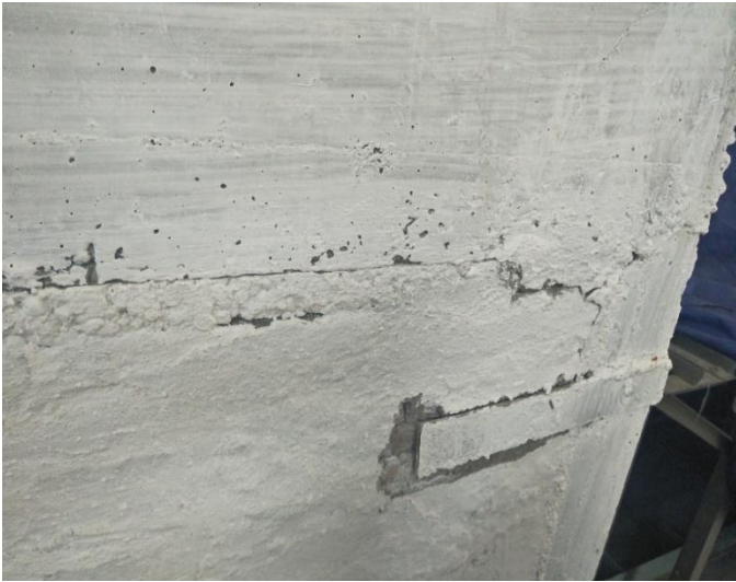
Figure 4: Cracks at 80% of NR1 (Styrofoam model)
