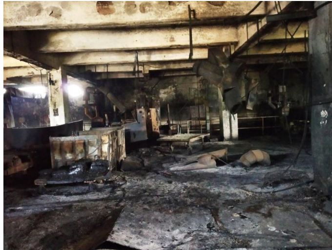
Figure 1: Interior view of first floor of damaged building
