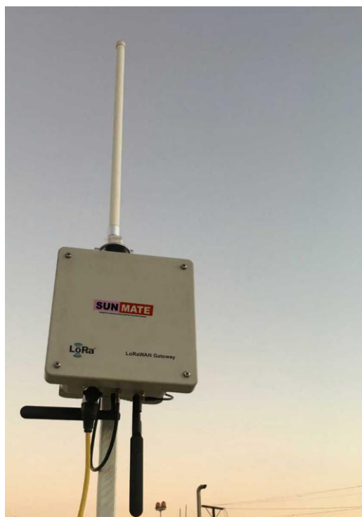
Fig.8: LoRa Gateway setup in Solar plant
