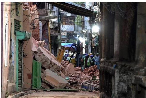
Fig.No.2 House Collapse during metro tunneling in Bow Bazaar, Kolkata (Google Source)
