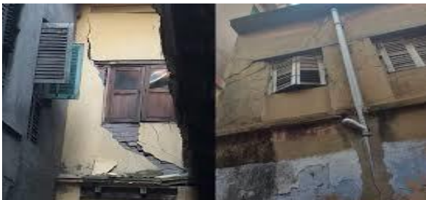
Fig. No.1 Homes emptied after cracks in Kolkata's Bowbazar (Google Source)
