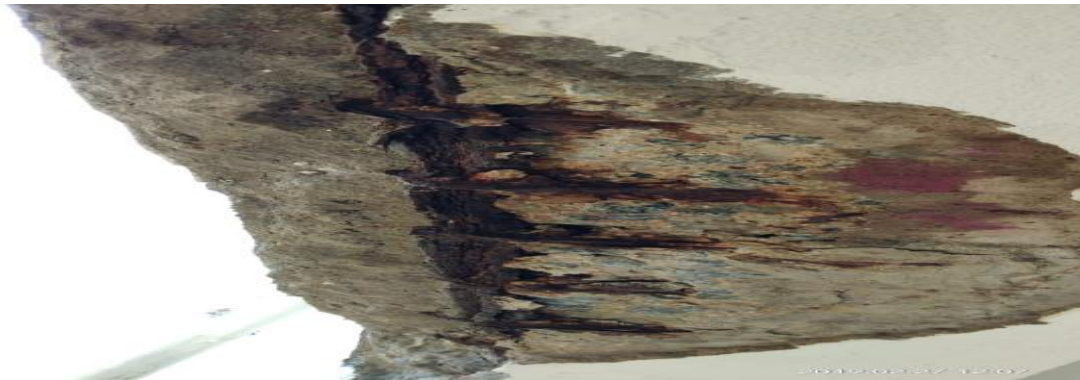
Fig 3.4 Applied phenolphthaleine indicator on a exposed reinforcement
