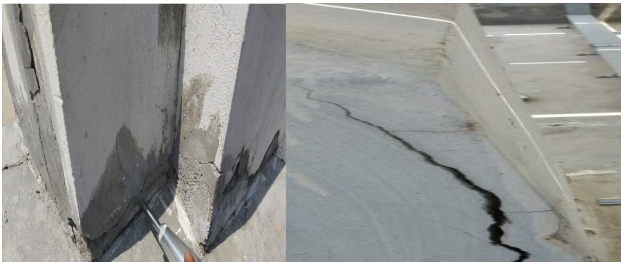
Fig .3.1 damages on a existing structure
