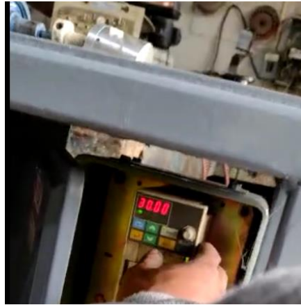
Figure 13: Set the speed on the variable frequency drive
