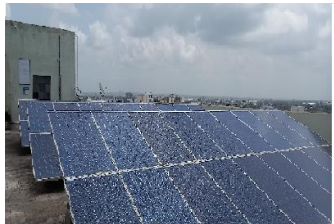
Fig 2 : Photograph of Solar Rooftop System
