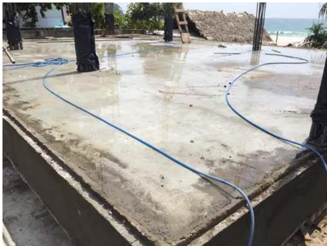
Fig - 1: Ponded concrete surface (Structural Guide 2021)
