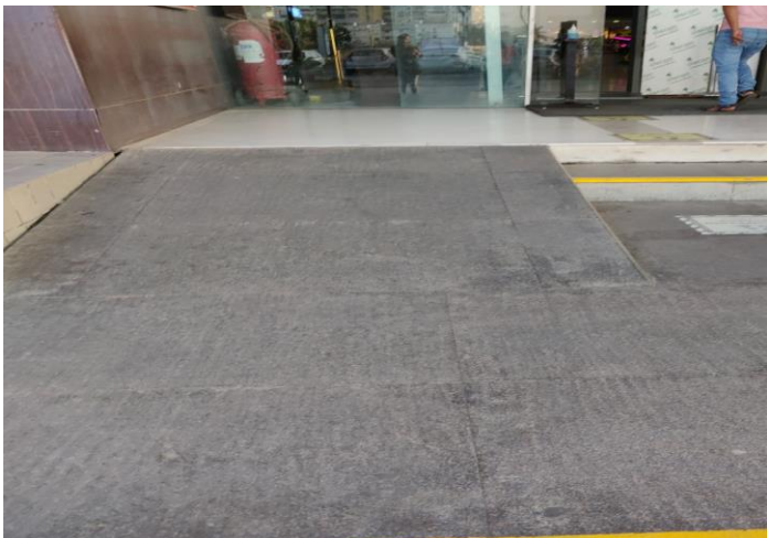
Fig-3 Ramp without handrail facility at Rahulraj mall
