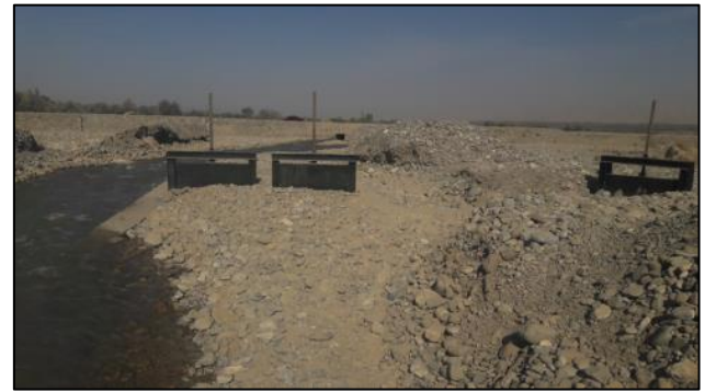
Figure 4: Damaged head works
