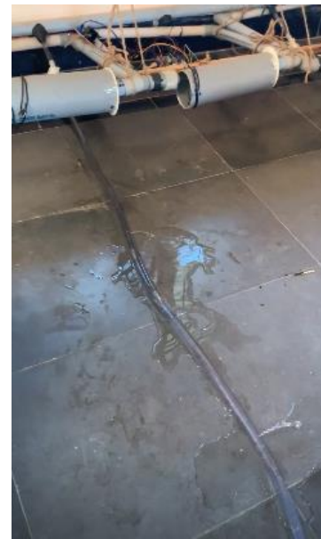
Fig: Water coming from slave pipe
