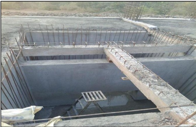
Fig 8 Problem- Plinth Beam passing through Septic Tank
