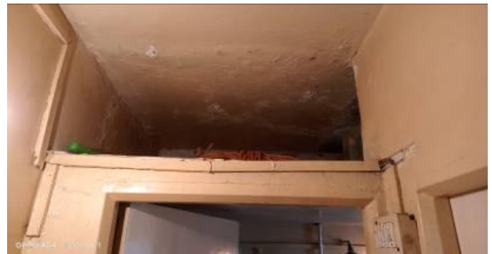
Image 2: Dampness and Colour Peeling in C1 06 flat
