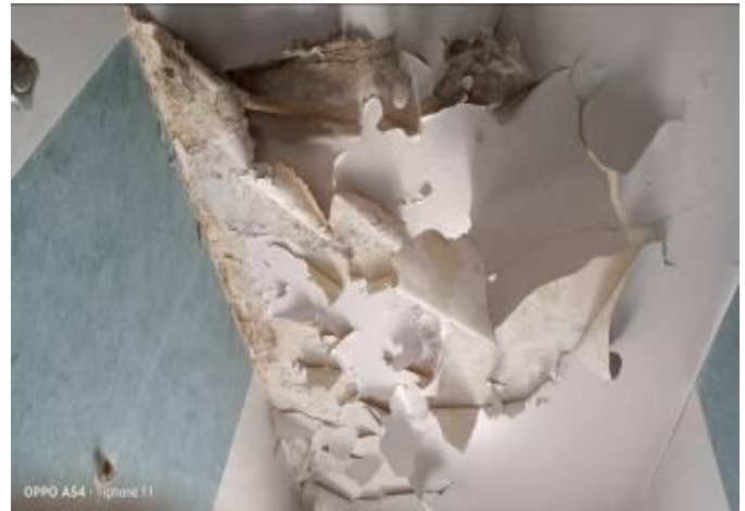
Image 1: Peeling of colour is observed at A-03 flat
