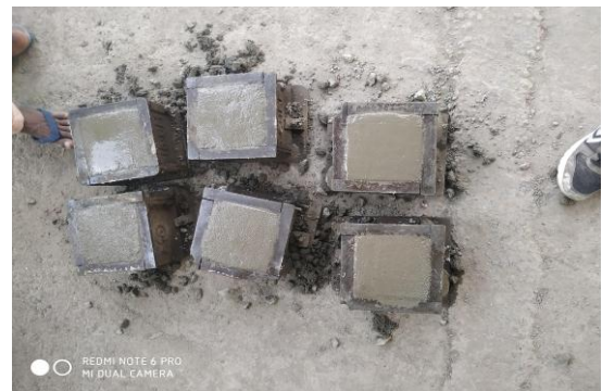
Fig- 4: Casting of specimen
