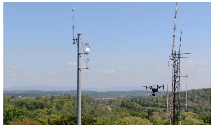
Fig. 10. UAS (drone) being used to confirm antenna alignment on Site B's radio towers (~85m height).
